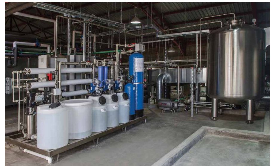
Water treatment and generation of purified water (PW), including water loop and storage tank
